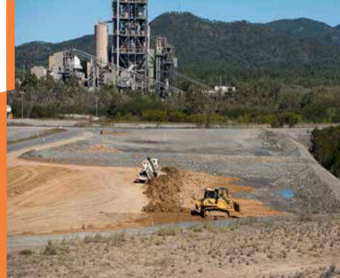
Earthworks to facilitate future port expansion on reclaimed land at Fisherman's Landing
