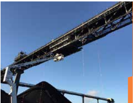
CC1A Gantry with access platforms and trolley
