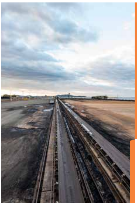
At Barney Point work continues to remediate the site and prepare it for bulk goods other than coal
