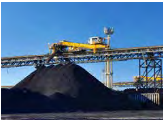
Unloading conveyor routes include a tripper, which travels along the conveyor and distributes the coal to the appropriate stockpile
