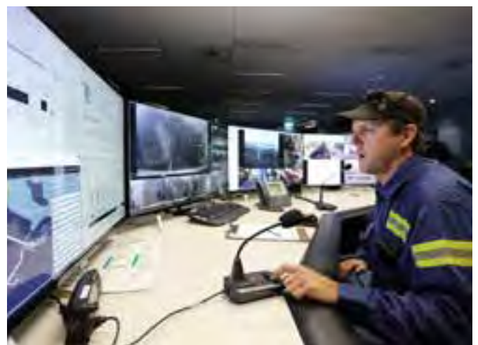
Since its commissioning in November 2016, there has been excellent operator acceptance of the new control system and control room
