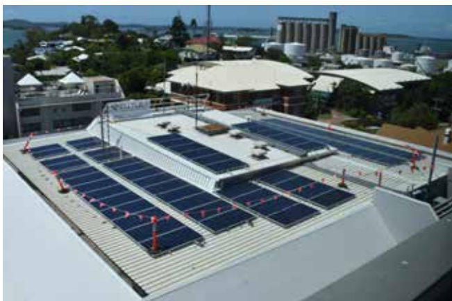
The solar panels installed are just the first step in GPC's solar power journey.
