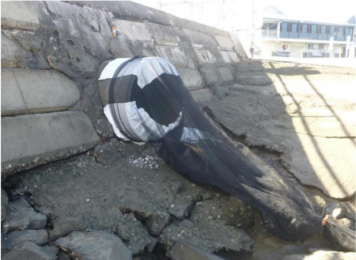
Figure 3. The tube net installed over the opening of the outfall pipe spilling into Auckland Creek, Gladstone (image: CQUniversity).
