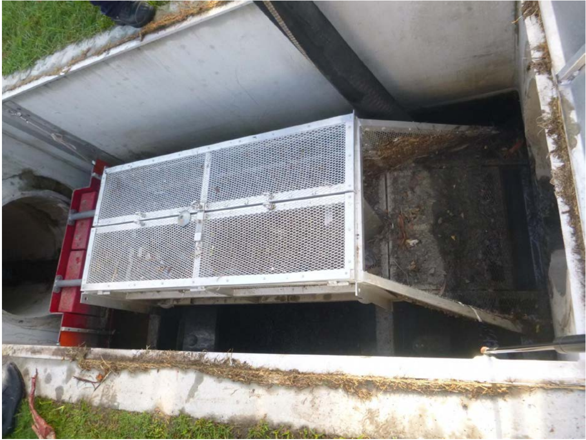
Figure 2. The SPEL Baffle Box gross pollutant trap installed at the corner of Goondoon Street and Lord Street, Gladstone (image: CQUniversity).
