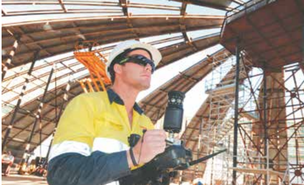
Construction progresses at the Queensland Curtis LNG site, July 2012. Photo courtesy of Bechtel Australia.
