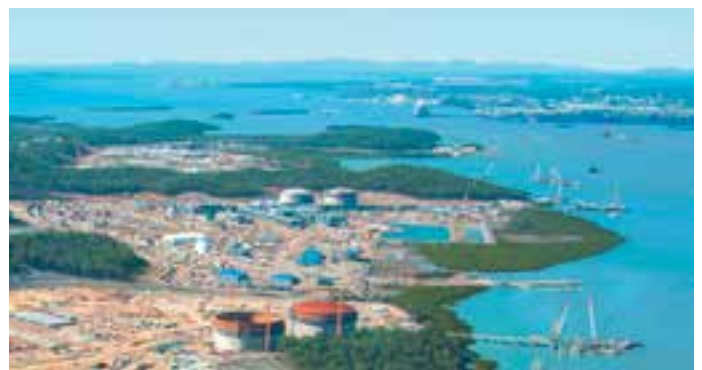
Three LNG processing plants were constructed on the southwest end of Curtis Island between 2010 and 2014.
