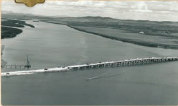
January 1966 - Construction of the William Barber Shaw Bridge. Photo courtesy of Queensland Alumina Limited.
