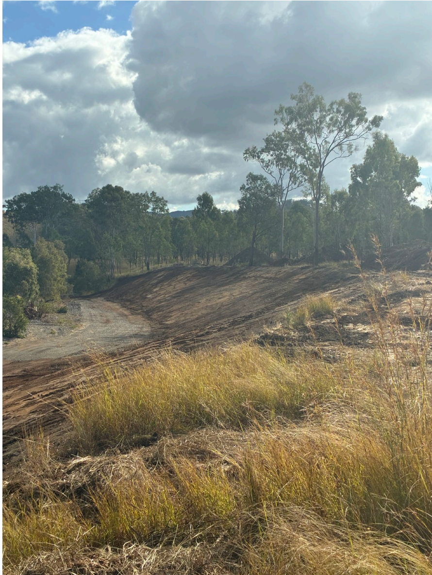
Figure 2. Progress image of site one. Reprofiling works have been completed as per designs. Image captured: 9 July 2025
